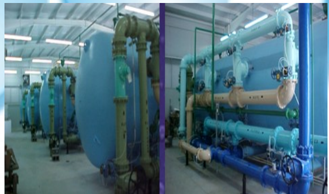
Brittany Drive Water Treatment Plant
